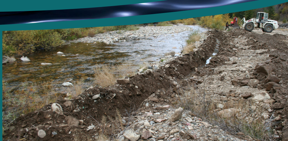
Left: Digging a trench at Pine Creek for riparian plants. Right: Camas plant often seen in wetland areas.
